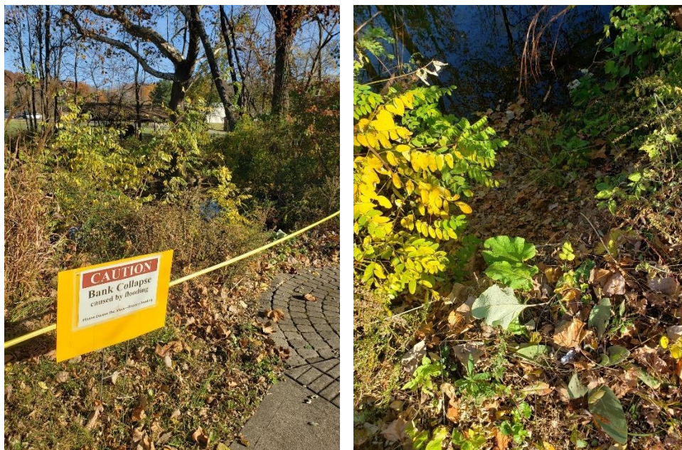
Figure 6: Bank collapse at Fetter's Run 2022
